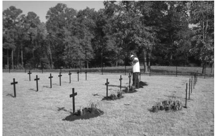
A worker erects one of 25 metal crosses the mark previously lost graves in the Old Gravel Point Cemetery in the Frierson community. The cemetery has been restored after being rediscovered during a pipeline crossing project last year. (Special to The Times)
