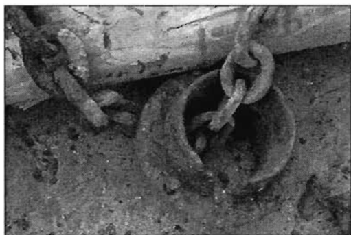
Figure 4. Anchor chain and through deck fitting.
