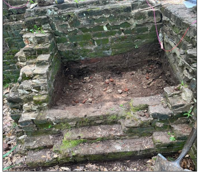
Figure 9. Inside wall of the kitchen area, presumably where a destructive fire started.
